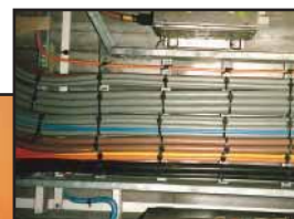
Marine Cable Bundling
